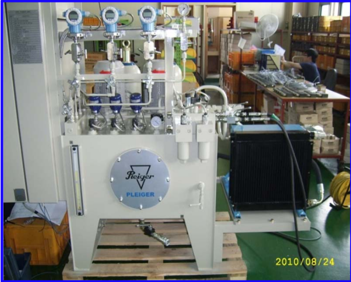
MAIN VALVE CONTROL HYDRAULIC POWER UNIT
